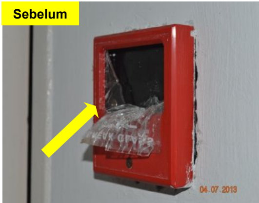
Gambar 1.50 Fire Break Glass Dirosakkan
